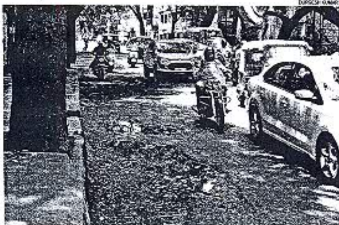
A pothole at Minerva Circle
